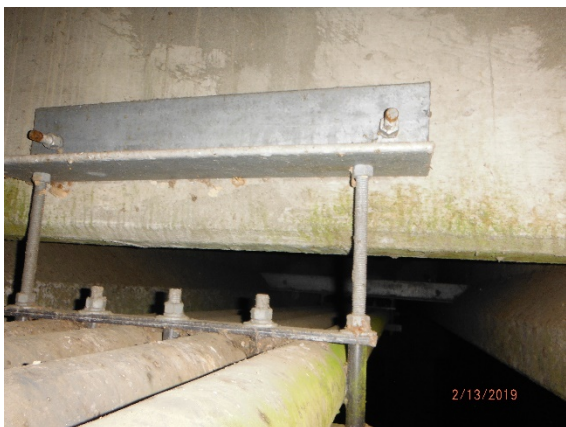
Photo 5. LBP Positive Pipe Support Channels
